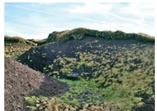
Figure 5: Gullies blocked by stone dams. These stabilise the gully floors, promoting re-vegetation and helping to raise water tables. Photo: © Moors for the Future.
