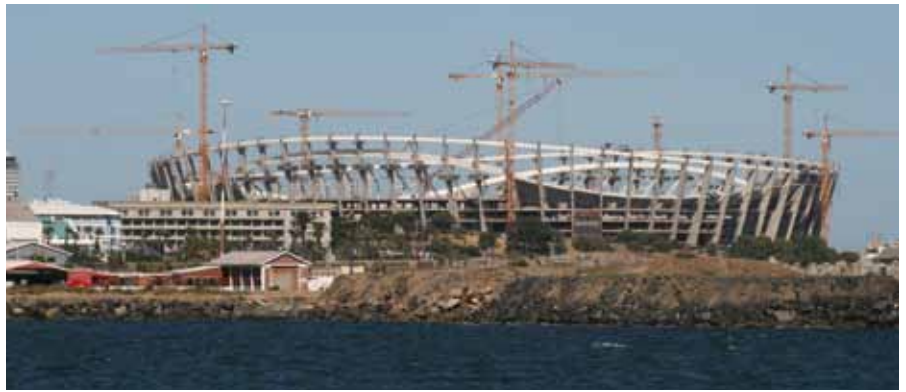
Green Point stadium under construction in Cape Town. Photo: Angus Willson/Tide~ global learning study visit.
